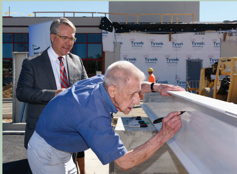
Lead donor James M Stockman signs a beam to be used in the construction the health system's new Cancer Institute that will bear his name.
